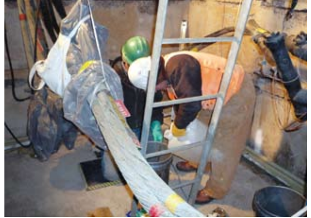
Jeff Kelly, NVE line working foreman, and Vic Camp, Voltek inspector, mixing up grout for the Voltek vault system track.
