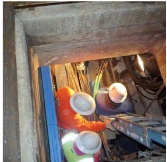
Material for the “vault-in-a-vault” solution was all lowered through the normal access door.
