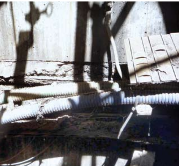
Degraded conditions in an underground vault required a creative fix.
